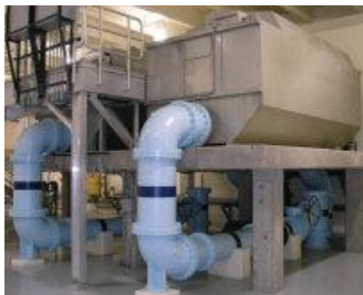
Hydrotech Discfilter Installation
