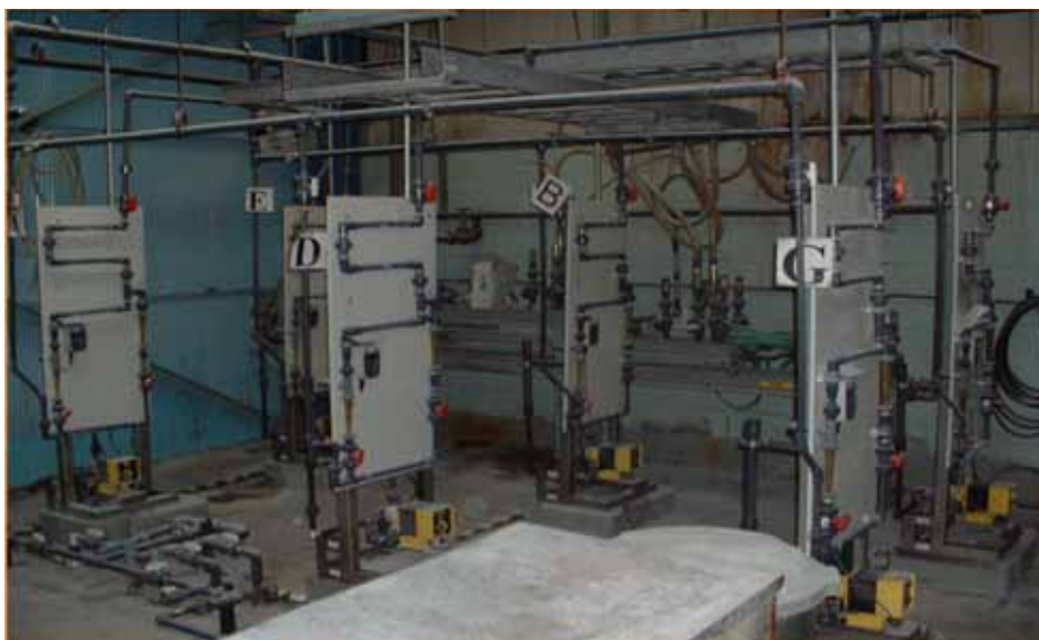
2001 Polymer Make-down utilizing LMI pumps and static mixers. The LMI pumps were replaced in 2002 with ProMinent Sigma 1 Control series pumps; control improved immediately.
