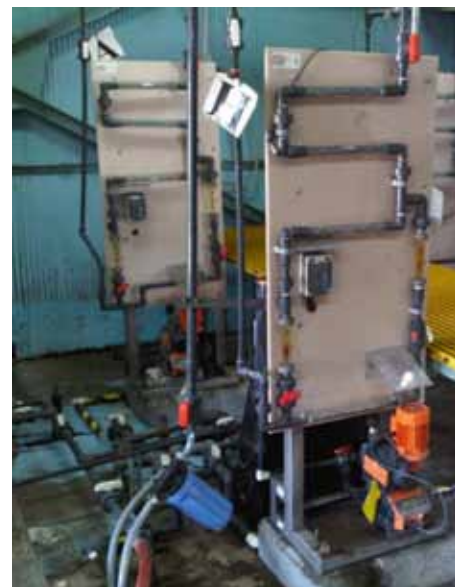
2002 Polymer Make-down system utilizing ProMinent Sigma pumps and static mixers.
