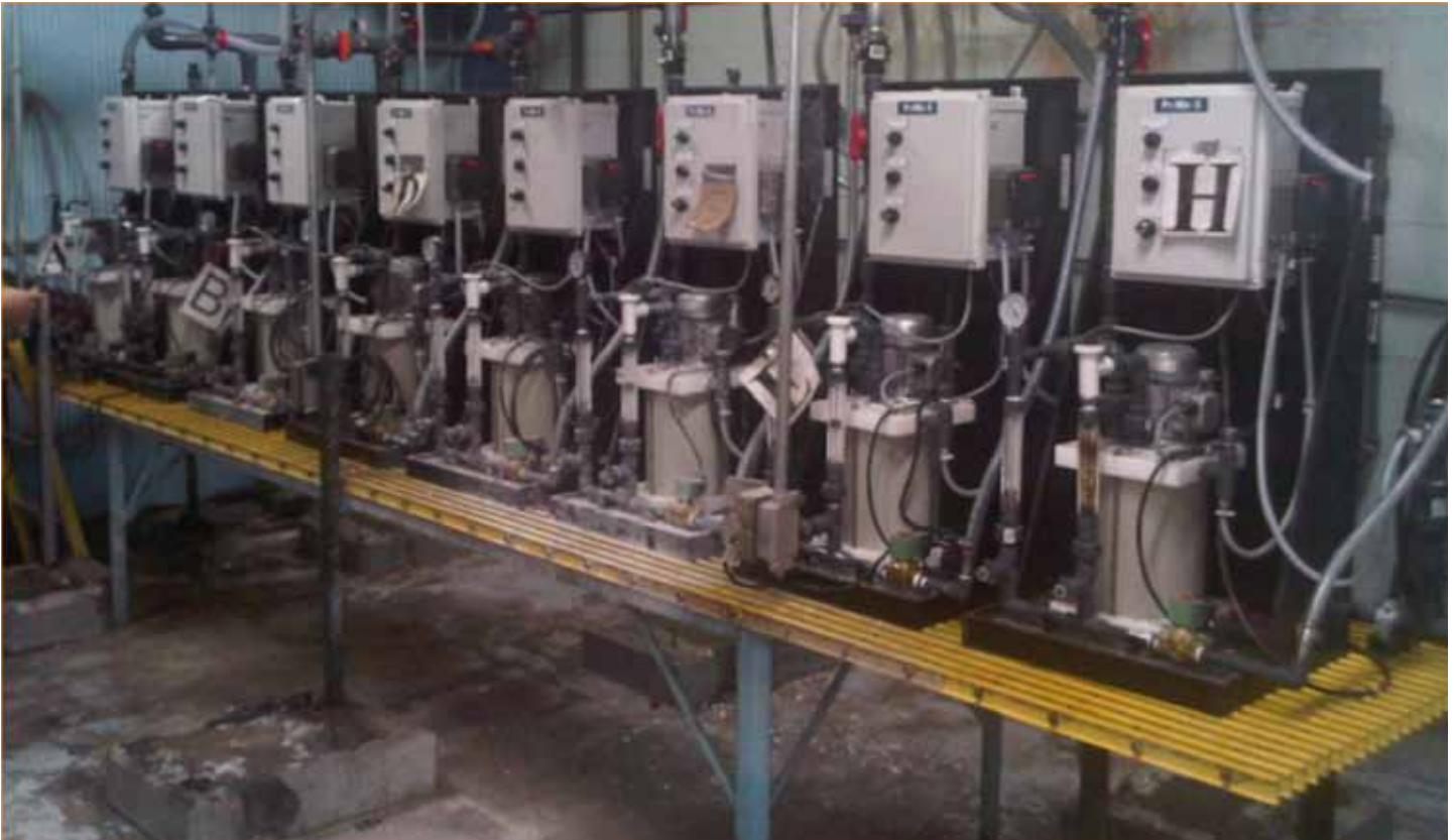
2010 completed installation and operational ProMix-S units.
