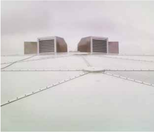
Dampers and louvers
